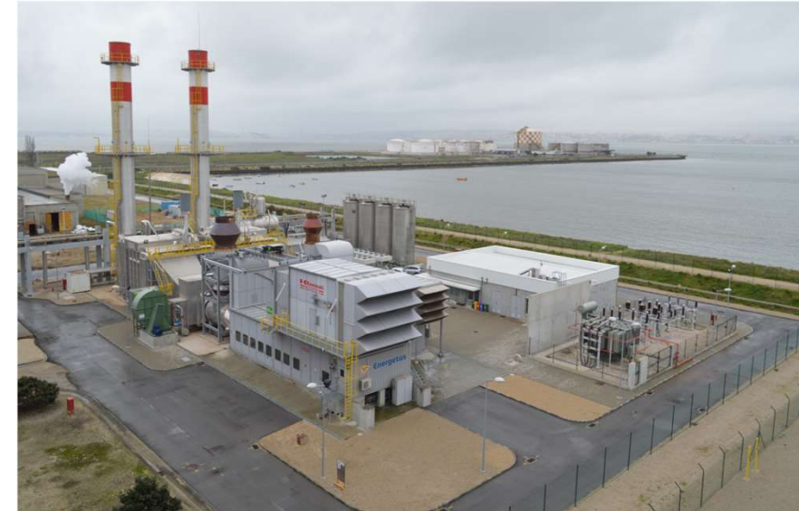
Barreiro power plant, 25 MW cogeneration
