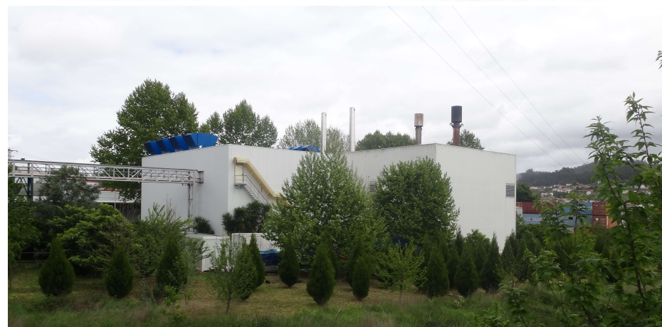
8,6 MW Gas Cogeneration Plant in Northern Portugal
